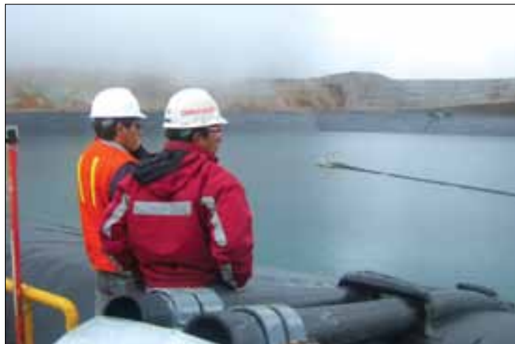
12" MINEFLEX on floating barge
