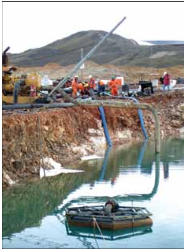
MINEFLEX on floating barge
