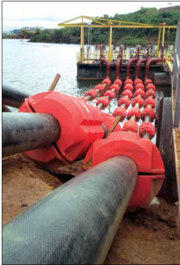
MINEFLEX on floating barge
