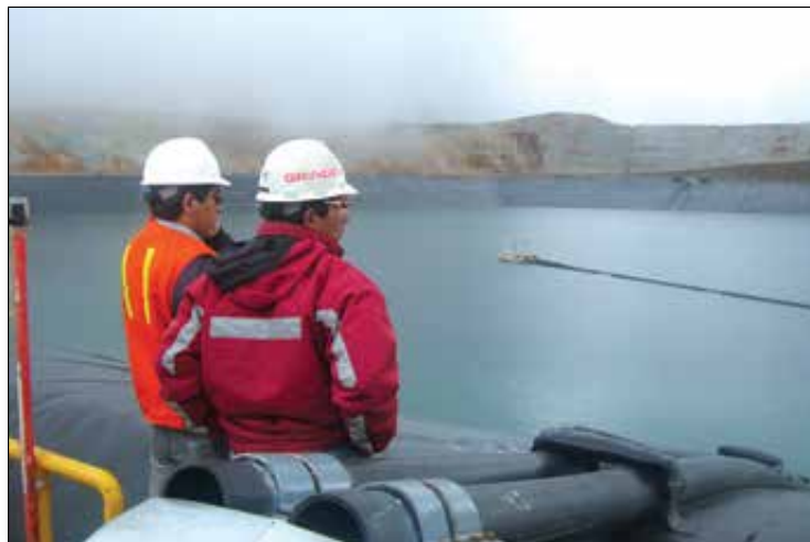
12" MINEFLEX on floating barge
